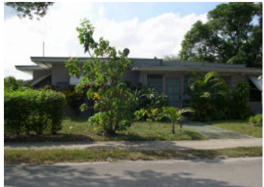
Rotting fascia; unkempt landscaping
