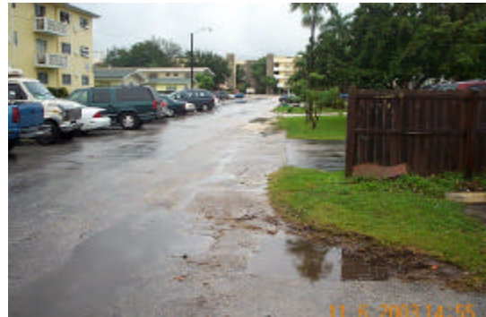
Missing sidewalks and storm drainage
