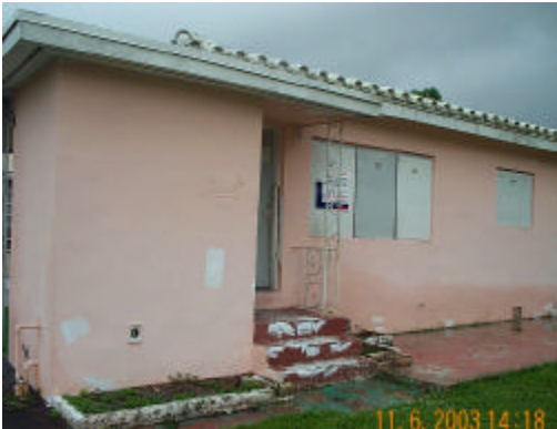
Peeling paint and plaster; broken steps
