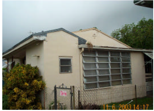
Rotting fascia; grass growing from roof
