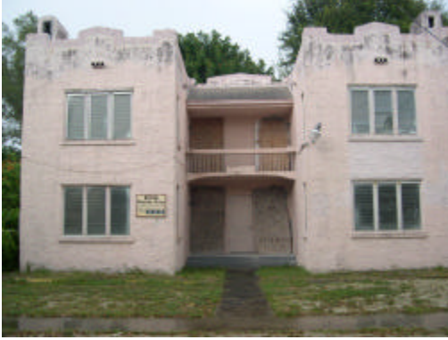
Unpainted; falling plaster
