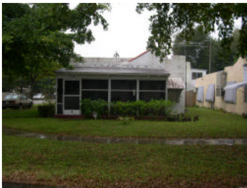
Lack of paint; broken screen
